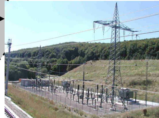
Power Supply System
