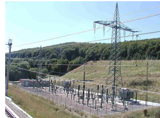
Power Supply System
