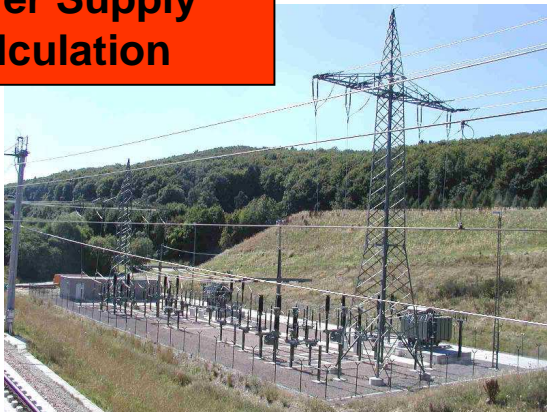
Power Supply System
